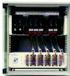
Emerson DeltaV Process Control System
