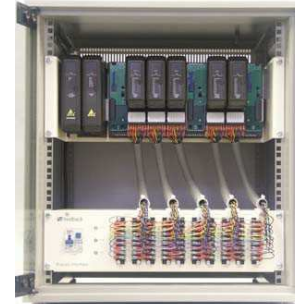
Control cabinet front view
